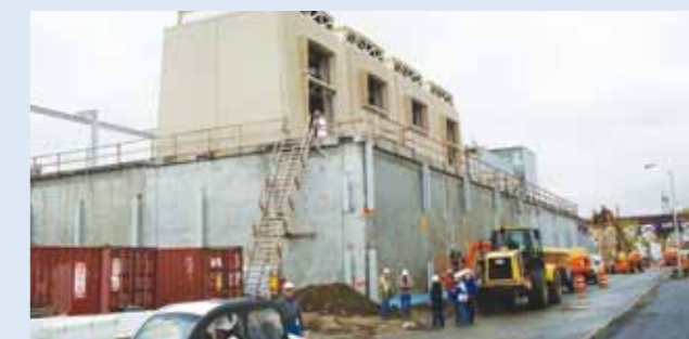
The United Utilities SHARON plant will provide a more environmentally friendly approach to treating liquors from sludge treatment
