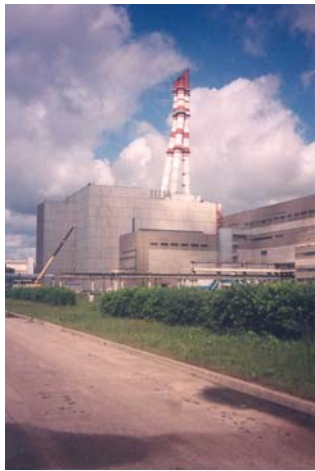
Ignalina Nuclear Power Plant - Decontaminating and dismantling of redundant equipment within Unit 1 Turbine Hall.
